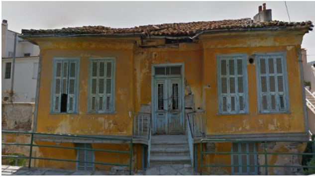
Figure 8. Two-Story Stone house on Th. Poulidou Street (Abandoned and Hazardous).
